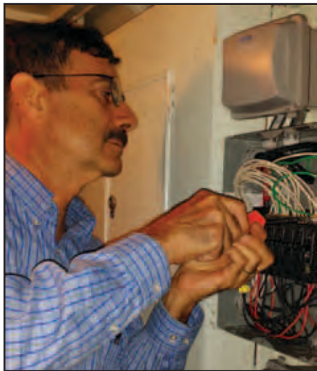
John LaCosta guided all of the electrical aspects of the generator and distribution system.
